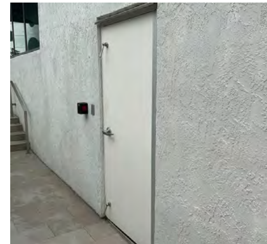
Permanent Flood Wall with Flood Door
