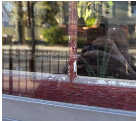
Figure 7 - Detail shot of typical condition of exterior paint on old windows.
