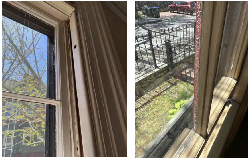
Figure 9 - Typical paint condition at older windows.
