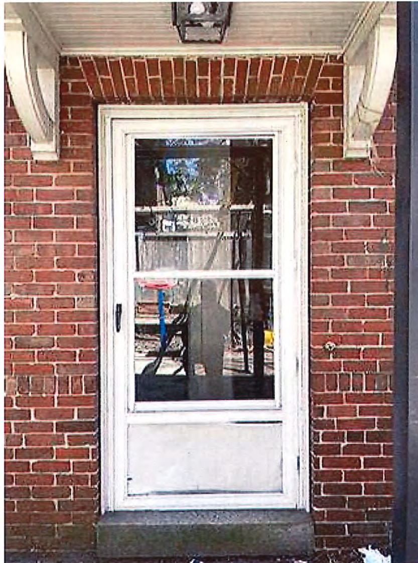
EXISTING NORTH (REAR) SIDE EXTERIOR STORM DOOR TO BE REPLACED WITH NEW STORM DOOR
