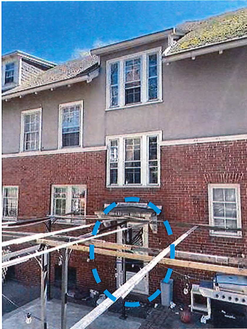
EXISTING NORTH (REAR) SIDE EXTERIOR STORM DOOR TO BE REPLACED WITH NEW STORM DOOR
