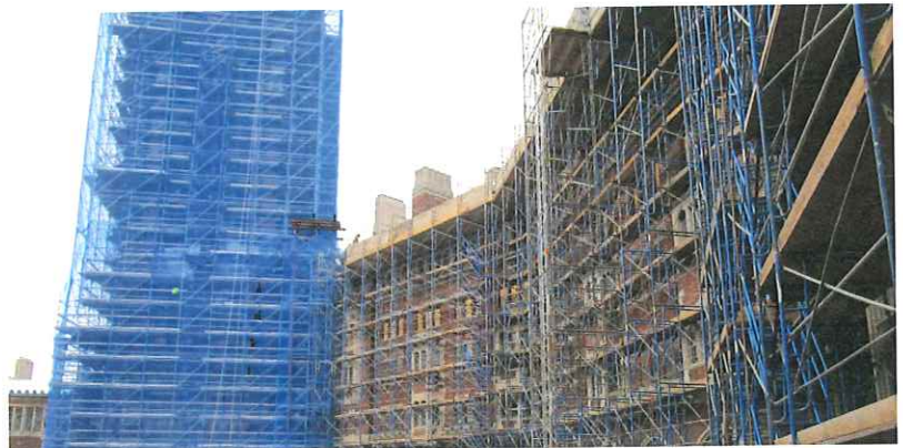
Project: Yale University 320 York Street Location: New Haven, CT Size: 5 building complex, 208,284 sf Completion Date: 2020 Client: Yale University Client Contact: James Elmasry, Yale University Senior Program Planner (203) 432-3875
