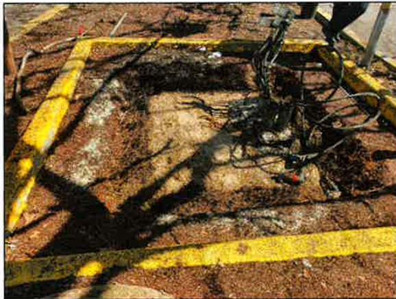
Photo 3 View of the Release Area subsequent to the removal of the concrete transformer pad, as viewed from the west.
