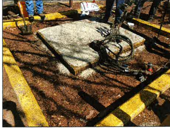
Photo 2 View of the Release Area during the performance of solid surface cleaning activities, as viewed from the southwest.
