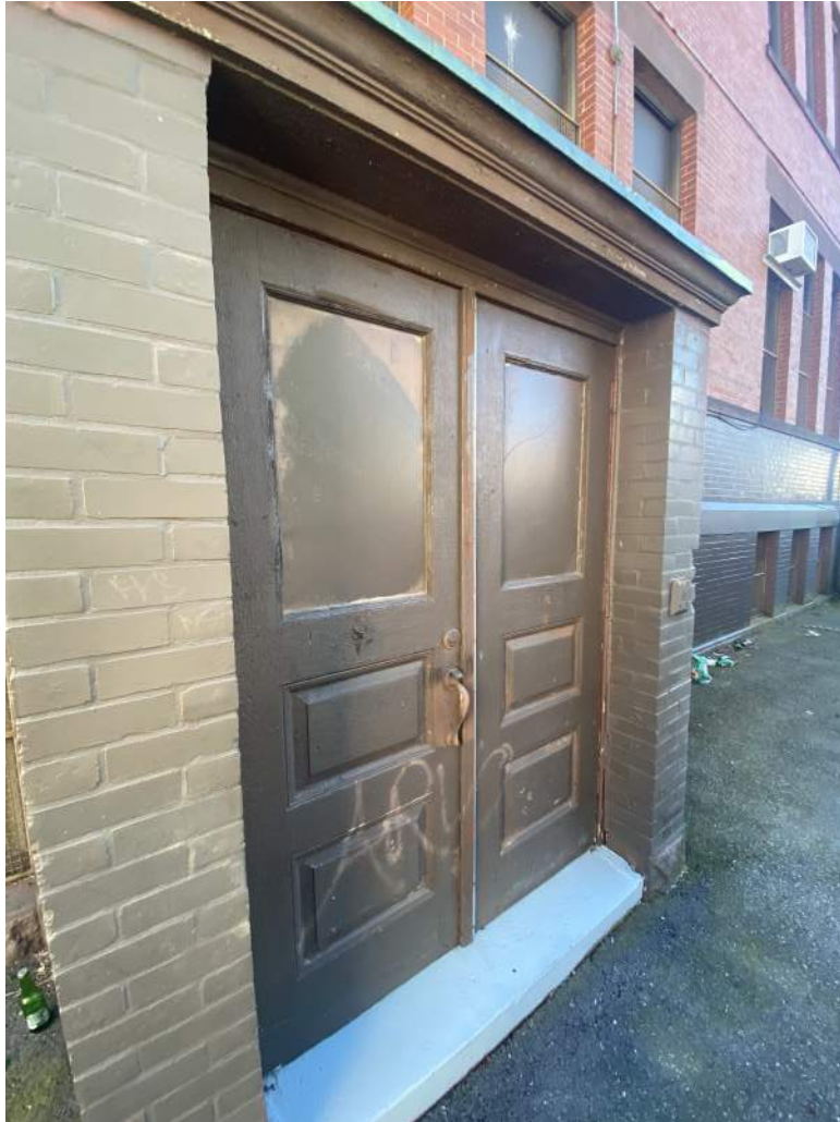
Photograph – 2: Photo depicts the typical application of asbestos caulk at window and door frames throughout the structure.
