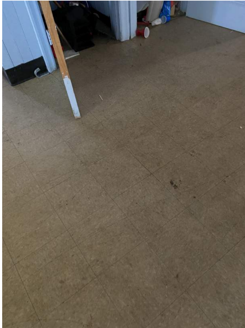
Photograph – 5: Photo depicts the typical application of asbestos vinyl flooring and associated glue throughout the structure, as scheduled for planned renovation.
