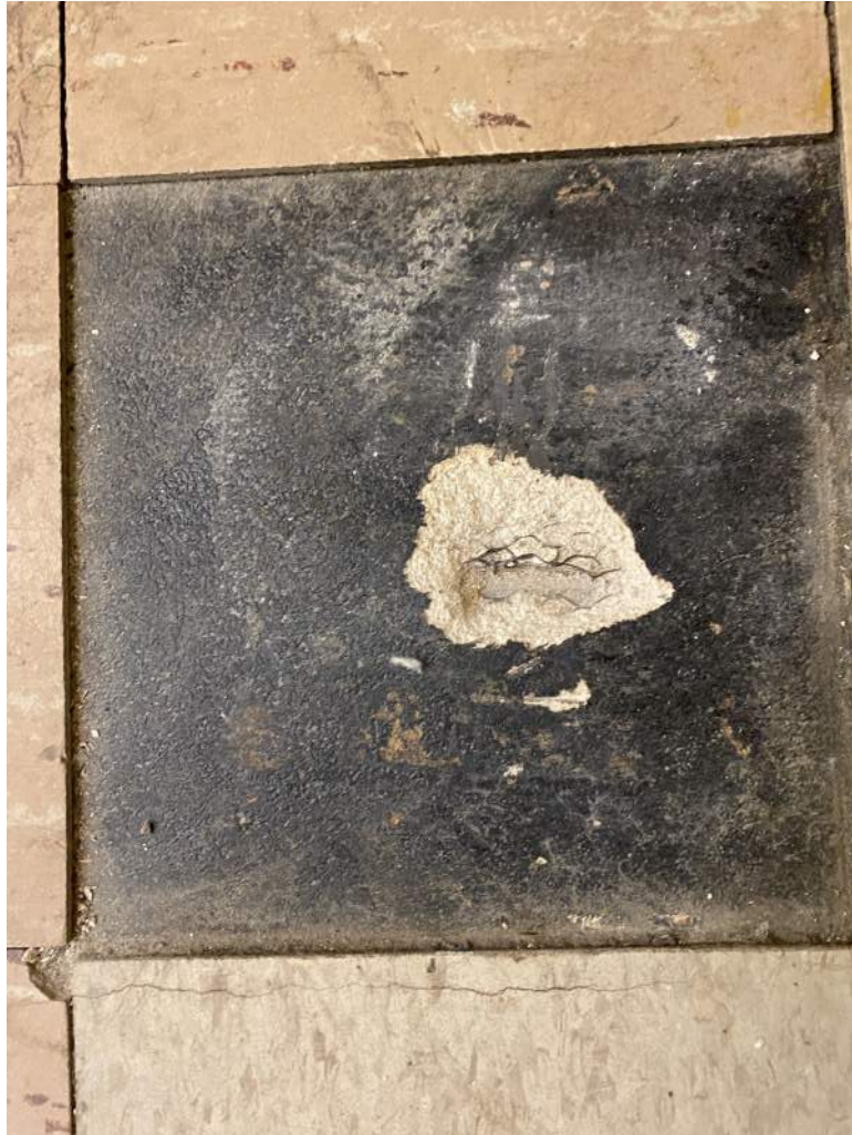
Photograph – 7: Photo depicts the typical application of asbestos concrete floor leveler existing or assumed to be existing at all floor surface areas throughout the structure, as scheduled for planned renovation.
