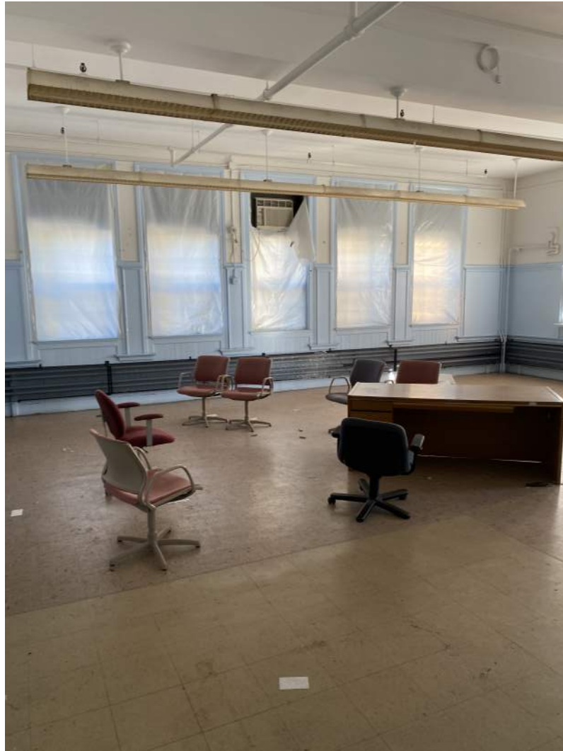
Photograph – 6: Photo depicts the typical application of asbestos vinyl flooring and associated glue throughout the structure, as scheduled for planned renovation.
