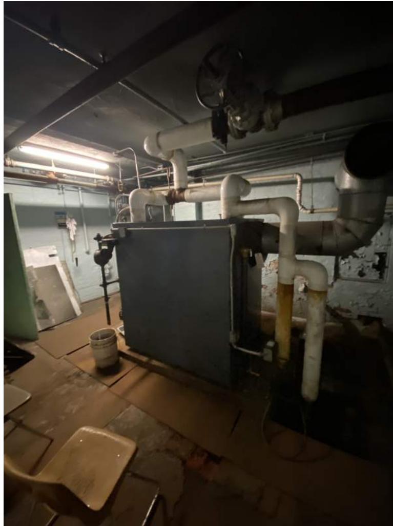
Photograph – 9: Photo depicts the existing boilers within the structure. These boilers are assumed to contain asbestos gasketing and packings. Additional investigation of the boilers should be conducted prior to removal.
