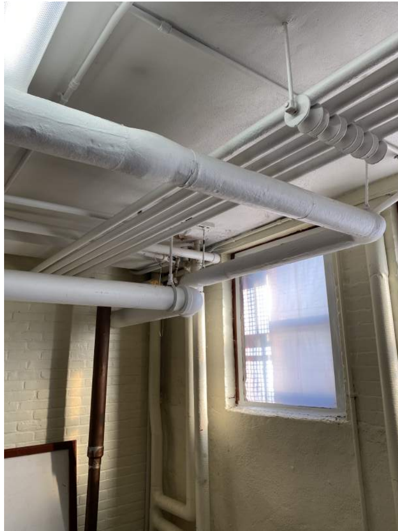
Photograph – 8: Photo depicts the typical application of asbestos thermal pipe insulation as applied to plumbing / heating systems throughout the Basement area of the structure, as scheduled for planned renovation.
