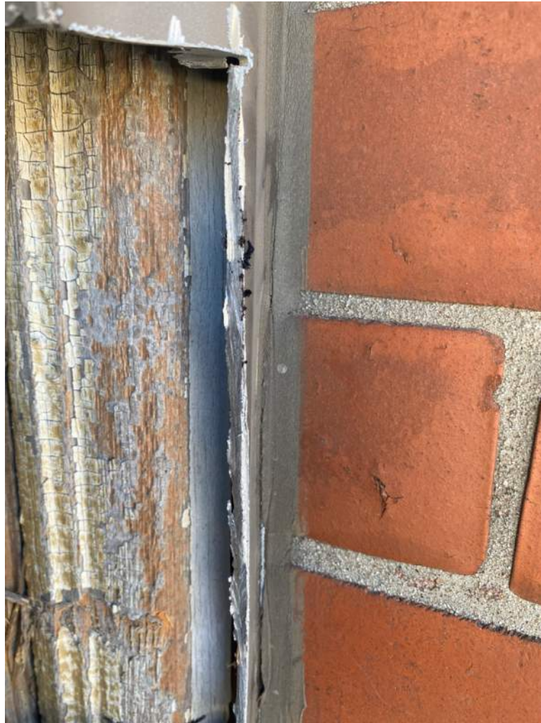
Photograph – 4: Photo depicts the typical application of asbestos caulk at window and door frames throughout the structure. Asbestos caulk is applied to the wood window frames enclosed behind the existing metal double hung windows. The removal of metal windows cannot be done without impact to the existing caulk at the wood window frames throughout
