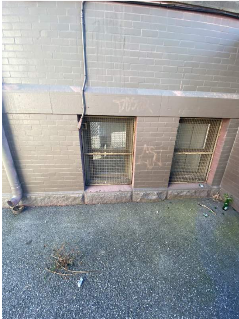
Photograph – 3: Photo depicts the typical application of asbestos caulk at window and door frames throughout the structure.
