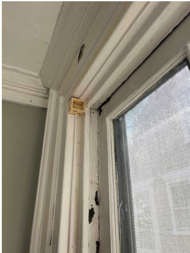
Figure 20 - detail of sash rubbing on frame
