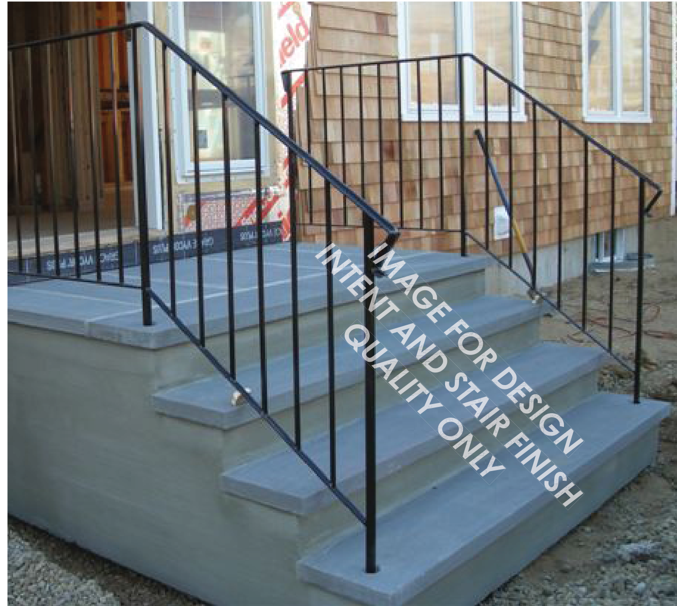
NEW BLUESTONE TREADS OVER EXISTING BROWNSTONE STEPS. INCLUDING REPAIR OF RISERS. TREAD AND RISER DIMENSIONS TO REMAIN CONSISTENT WITH EXISTING CONDITIONS.
