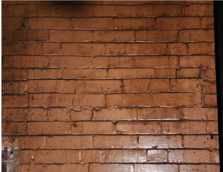
Interior painted brick shaft. Paint is positive as LBP.
