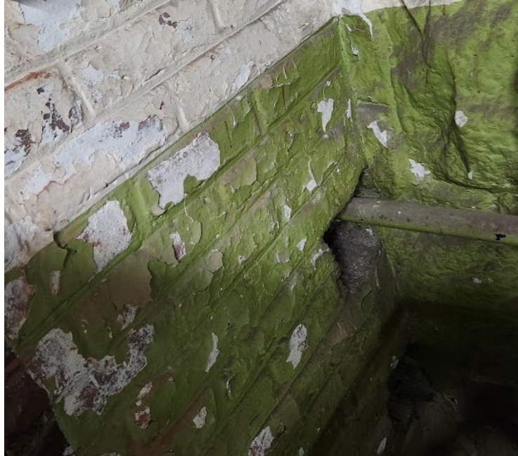
White and Green basement paint identified as LBP.
