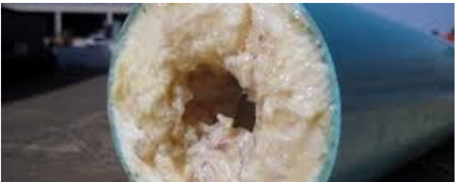
CLOGGED PIPE WITH FOG
