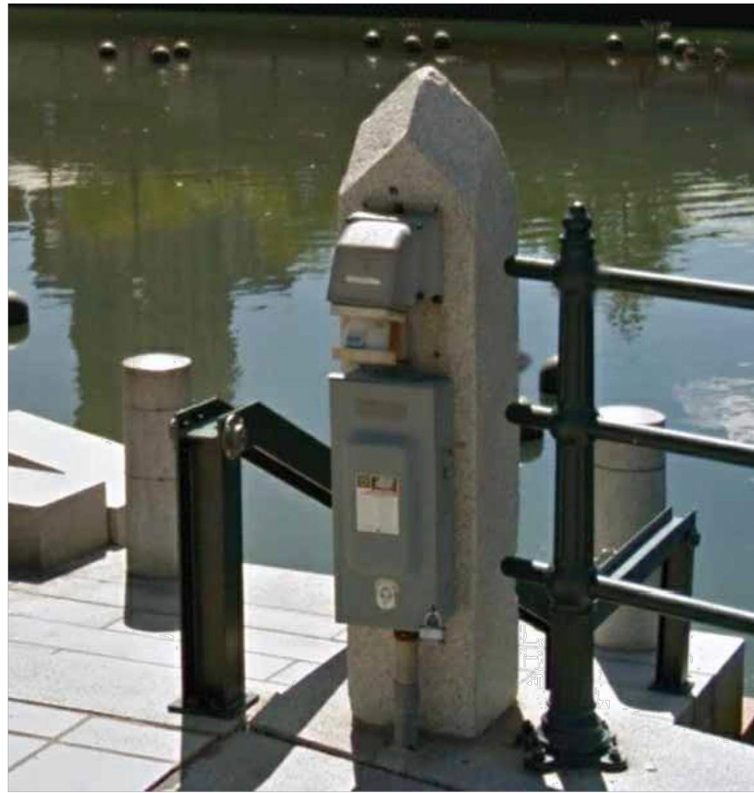
PHOTO OF EXISTING PIN AND SLEEVE RECEPTACLE
