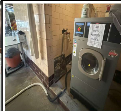
PHOTO 7: WASHING MACHINE DRAIN WITH HOSE RUNNING ACROSS FLOOR
